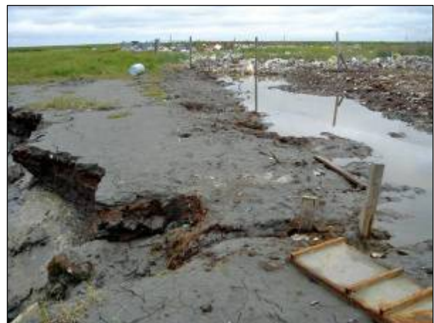
Eroding riverbank next to Kwigillingok's dump.
