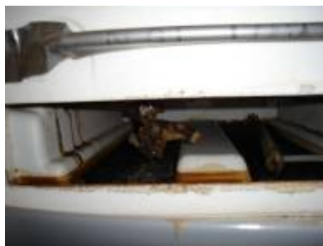
Figure 98: Bottom of the store toilet while emptying (panel and tray removed, and looking in).
