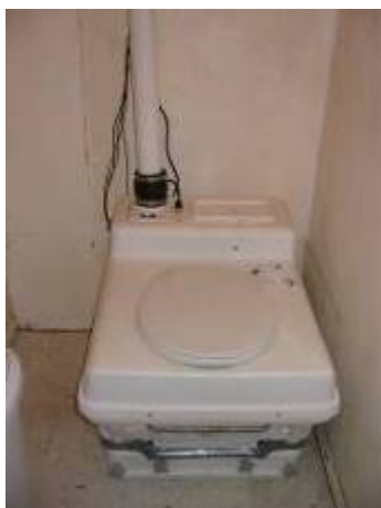
Fig 55: Compost toilet positioned in bathroom with (white) vent pipe and sensor wires in place
