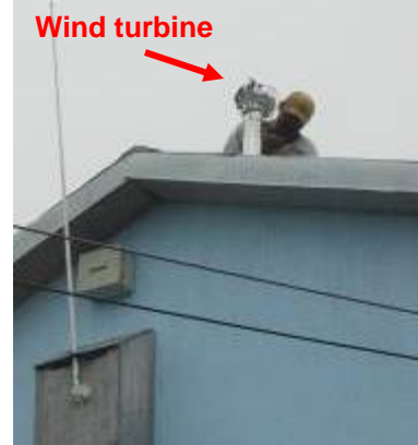
Fig 61: Wind turbine being placed on top of the aluminum insulated vent pipe for the store toilet
