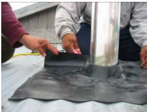
Fig 85: Setting the roof flashing to lie flat and secure on the roof.
