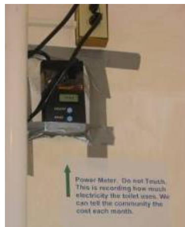
Fig 71: Sign explaining to the public about the power meter attached to the wall
