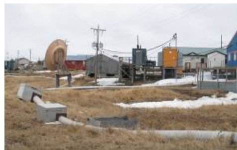
Figure 19: Wastewater piping from the school to the separate school lagoon
