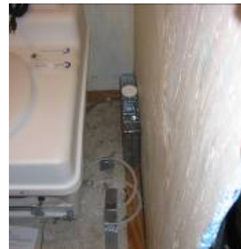
Figure 44: Water container and modified drain pipe connected to the Envirolet
