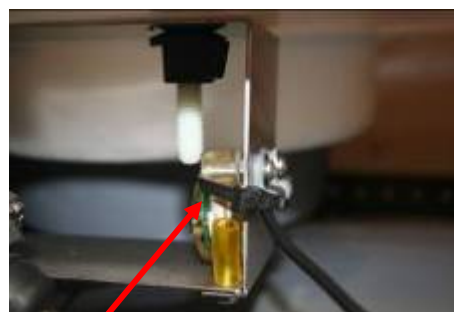
Figure 32: Tidbit backup temperature sensor
