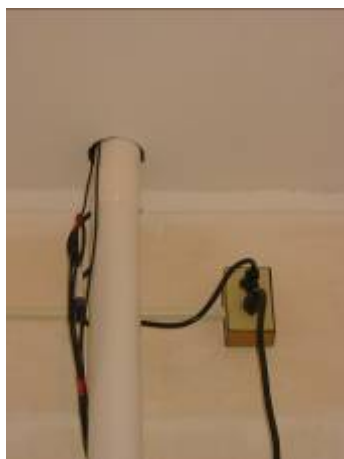
Fig 56: Vent pipe exiting through the bathroom ceiling into the attic with sensor wires running by the side of the pipe
