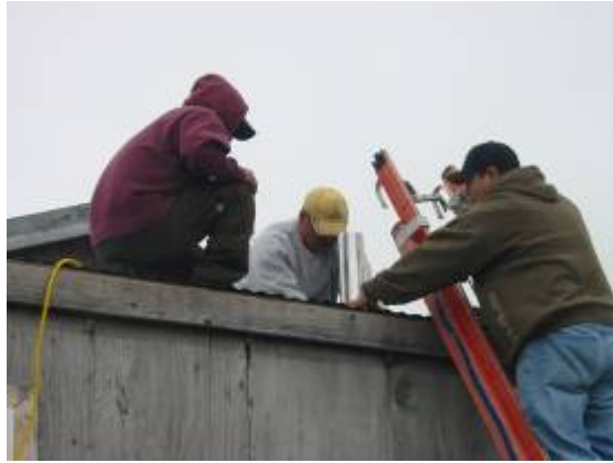
Fig 82: Fitting the aluminum insulated section to the top of the vent pipe.
