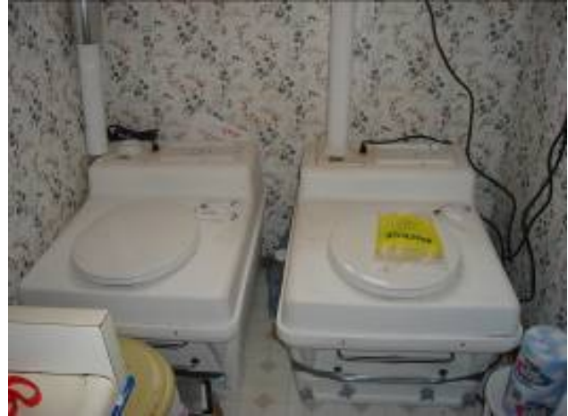
Fig 93: Toilets A and B set in place in the Moss's bathroom, against the back wall, for installation.
