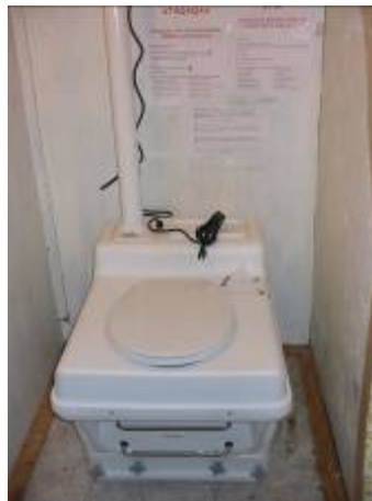
Fig 88: Installed toilet at the Tundra's with signs up on the back bathroom wall.
