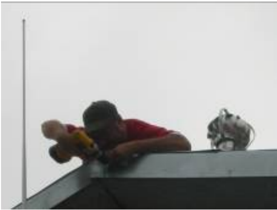
Fig 62: Close-up of the satellite antenna mounted to the roof
