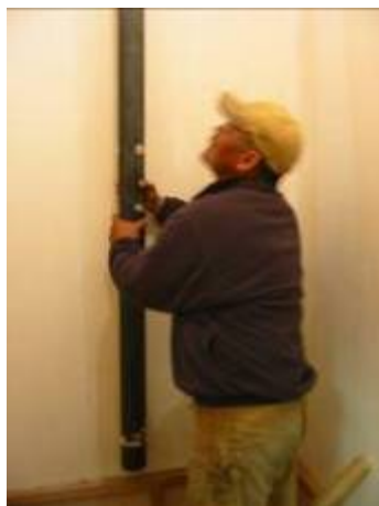
Fig 53: Taking out the existing (black) vent pipe in the store bathroom for compost toilet installation preparation
