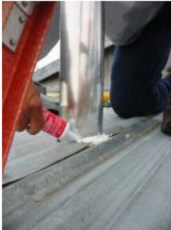
Fig 83: Using silicone sealant to fill any gaps at the vent pipe outlet.
