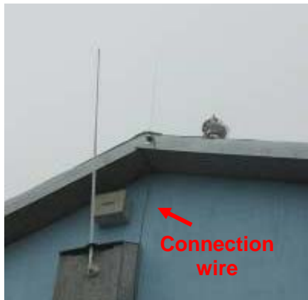
Fig 64: Satellite antenna with the connection wire leading down to the attic space where the data transceiver was located
