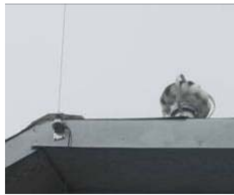
Figure 39: Close-up of the installed antenna on the roof
