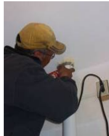
Fig 65: Sealing the air gaps at the vent pipe outlet in the bathroom ceiling with silicone sealant
