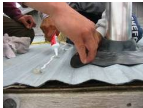
Fig 86: Using silicone sealant to secure the roof flashing to the corrugated metal roof for weatherproofing.
