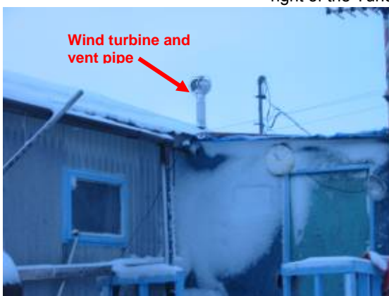
Fig 91: Wind turbine and vent pipe above the bathroom at the Tundra's household. Photo taken in the winter, four months after the Tundra's toilet was installed.
