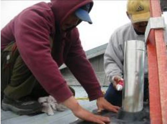
Fig 60: Aluminum insulated vent pipe section above the roof line, and rubber flashing being sealed to the roof
