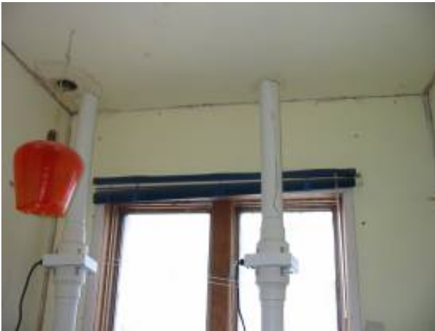
Fig 94: Vent pipes with turbo fans being set into holes drilled in the ceiling for Toilets A and B in the Moss's bathroom.
